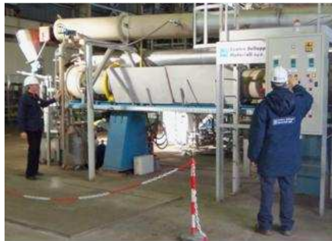
CSM 120 kW Pilot Plant
